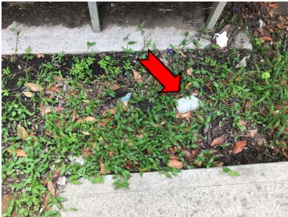
Photo 3. Exterior, throughout, ground – asbestos-containing fibre cement debris.
