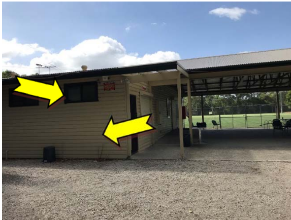
Photo 9. Exterior, throughout, walls and features – suspected lead-containing yellow and green upper coloured paint systems.
