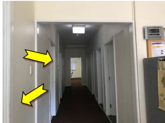
Photo 10. Interior, throughout, walls and door frames – suspected lead-containing light yellow and white upper coloured paint systems.
