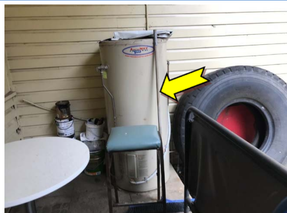
Photo 6. Exterior, south-west elevation, hot water heater – suspected SMF internal insulation material.
