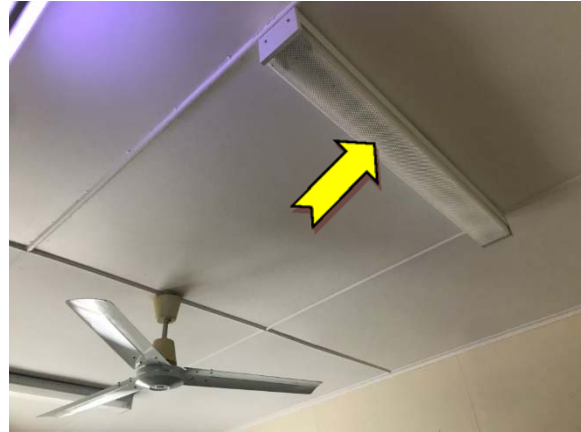
Photo 8. Interior, throughout, fluorescent double tubed light fitting – suspected non PCB-containing capacitors.
