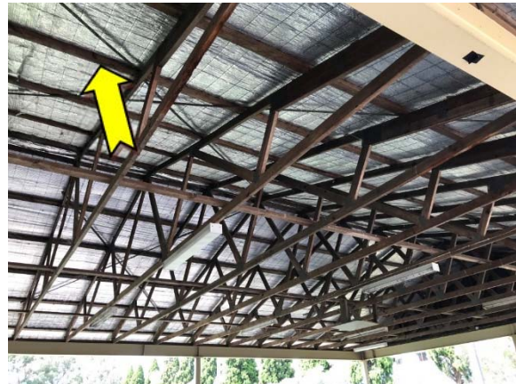
Photo 4. Exterior, south-east elevation, underside of awning – suspected SMF sarking insulation material.
