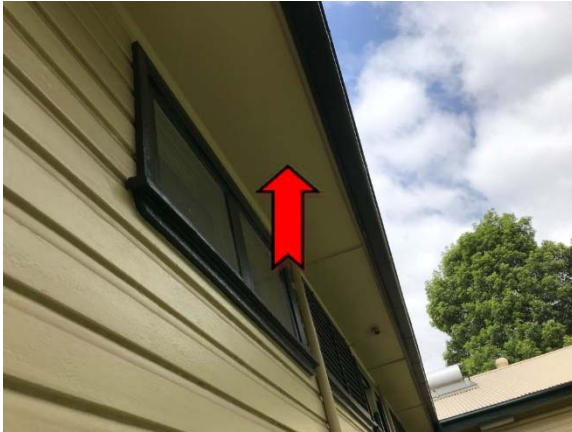
Photo 1. Exterior, throughout, eaves – asbestos-containing fibre cement sheeting.
